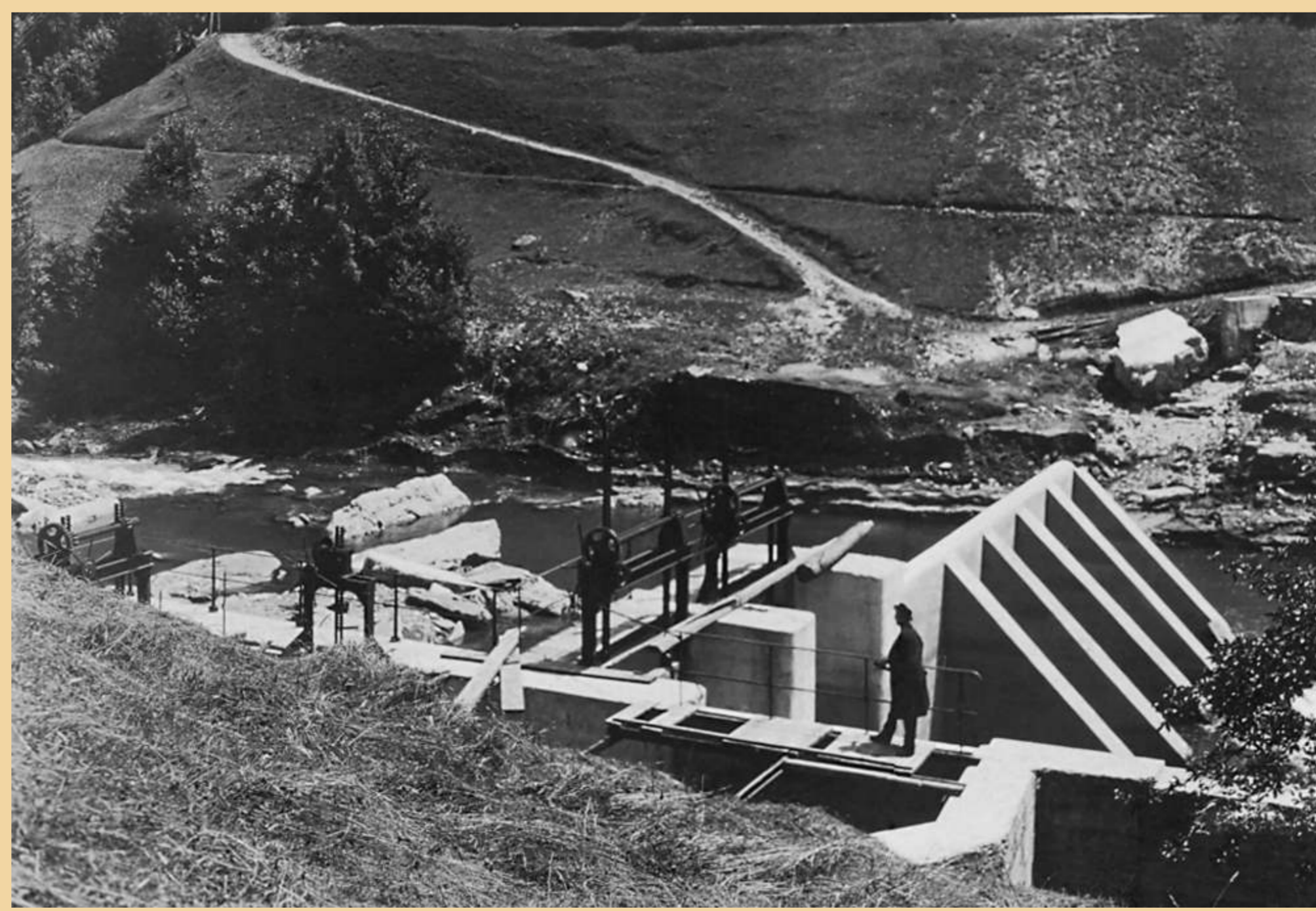
[11] Podrt jez žirovske elektrarne na Fužinah, po povodnji leta 1925, slikano z levega brega Sore. Ruined dam of the Žiri electric power plant at Fužine after the flood of 1925, as seen from the left bank of the Sora River.
