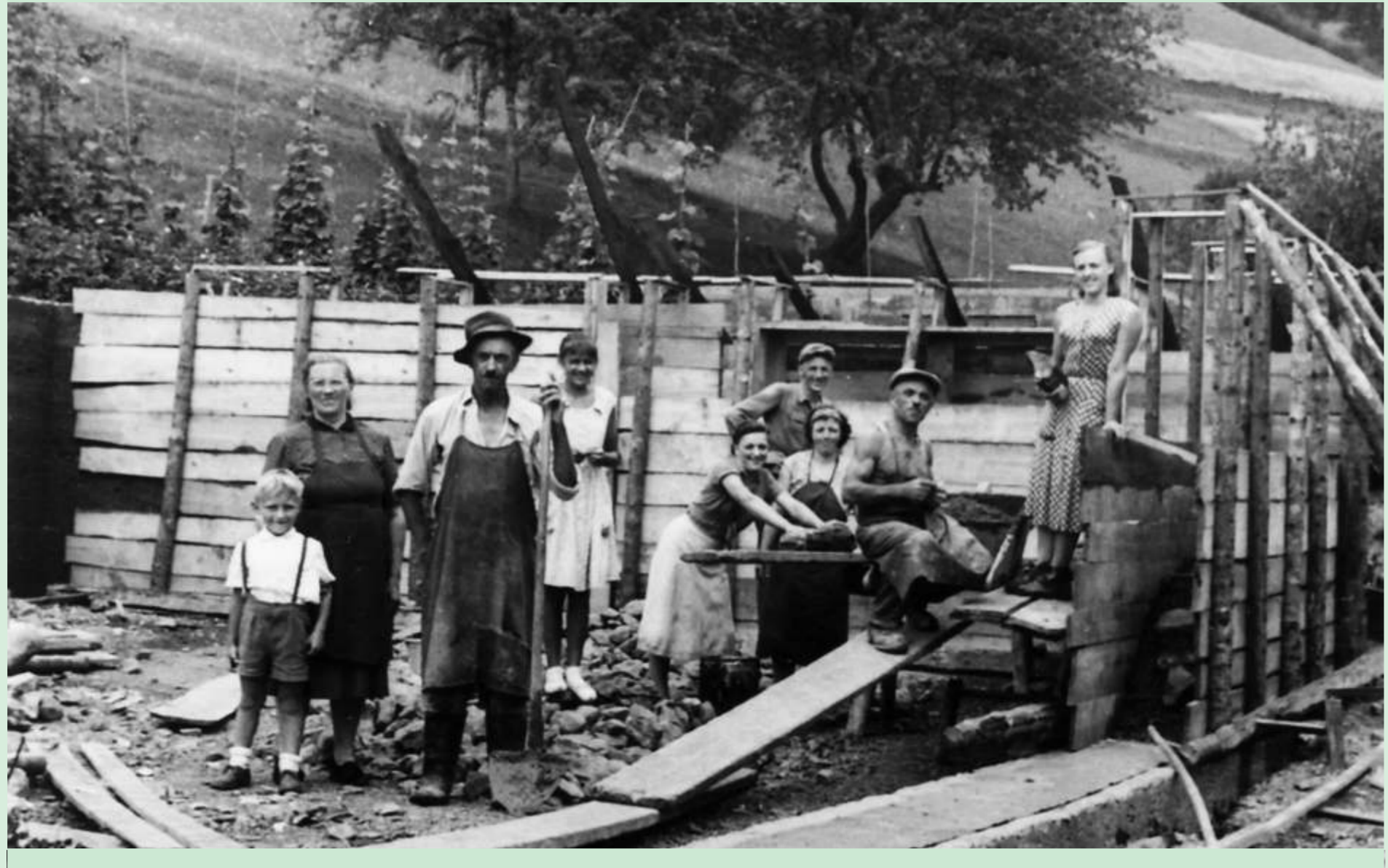
Tako so naredili opaž za betoniranje pritličnega dela nove hiše Bogdana in Tončke Cankar. Z leve: mali Mirko, stara mama Malka, Jakob Žakelj – Črvov, Stanko Capuder, Hilda Miklavčič, Tončka Cankar, ata Franc Miklavčič, Anica Miklavčič, zadaj Bogdan Cankar. Selo, 19. julij 1959. This is how panelling was made for concreting the ground floor of a new house.
